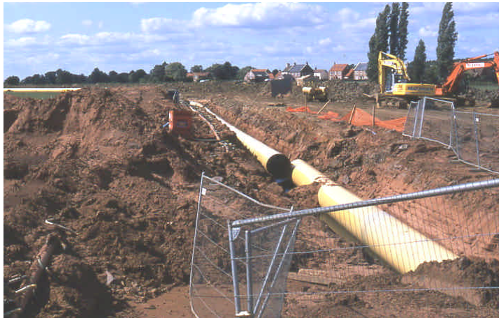
Fig 3.4.2 Gas pipeline being laid South of Gateforth village. Heavy equipment being used.
